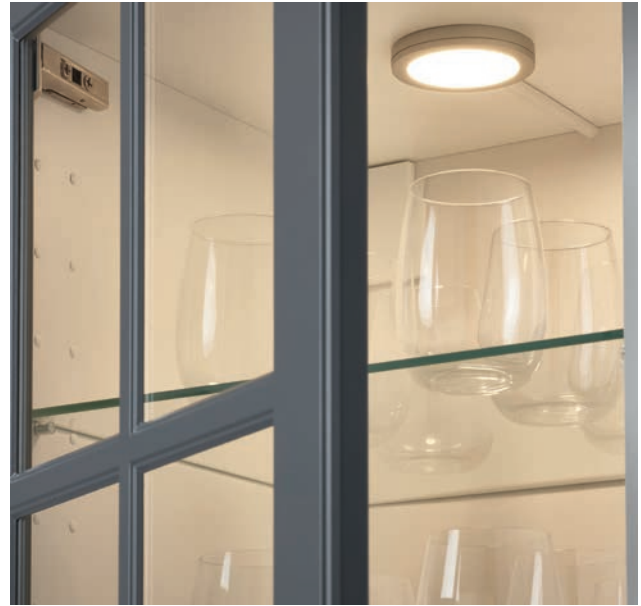
Spotlight in cabinet
