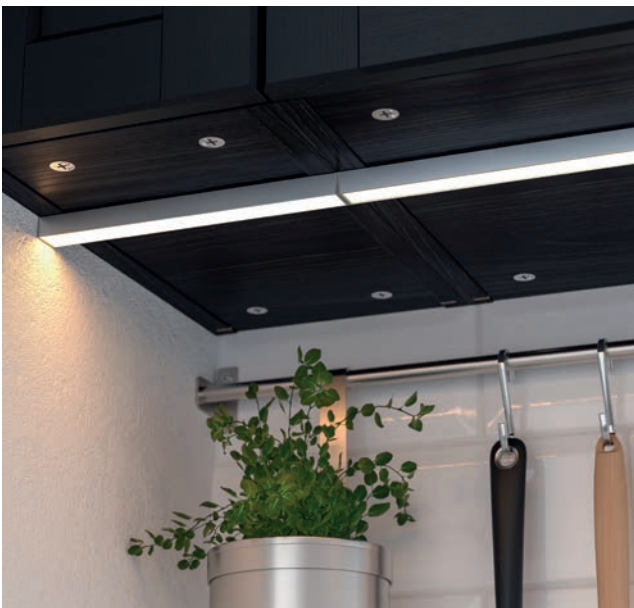
Lighting strip under wall cabinet
